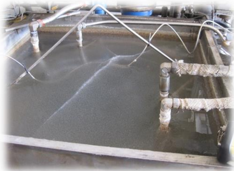
Heat exchanger tank frozen over
