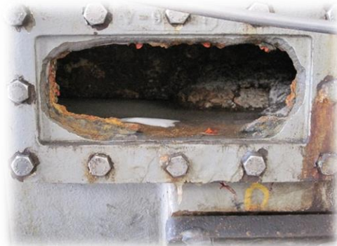
Water jacket cover destroyed by ice.
