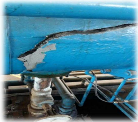
Cracked cylinder water jacket
